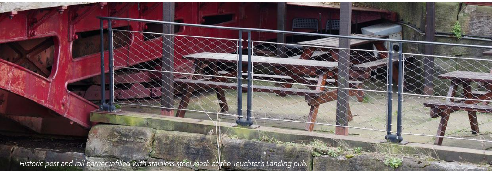
Existing barriers around Albert Dock including timber palisade fencing and armco barriers.
